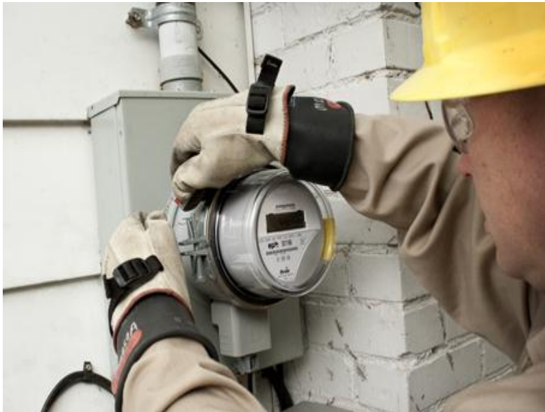
An employee installs a smart meter as part of a smart grid initiative by EPB. The project is supporting 390 jobs in the Chattanooga area. | Photo courtesy of EPB
